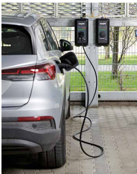
Charging stations of SWM.
