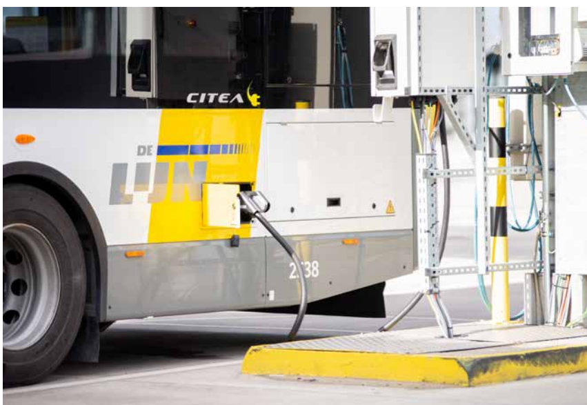
PSI's depot and charging management system controls the E-buses at De Lijn.
