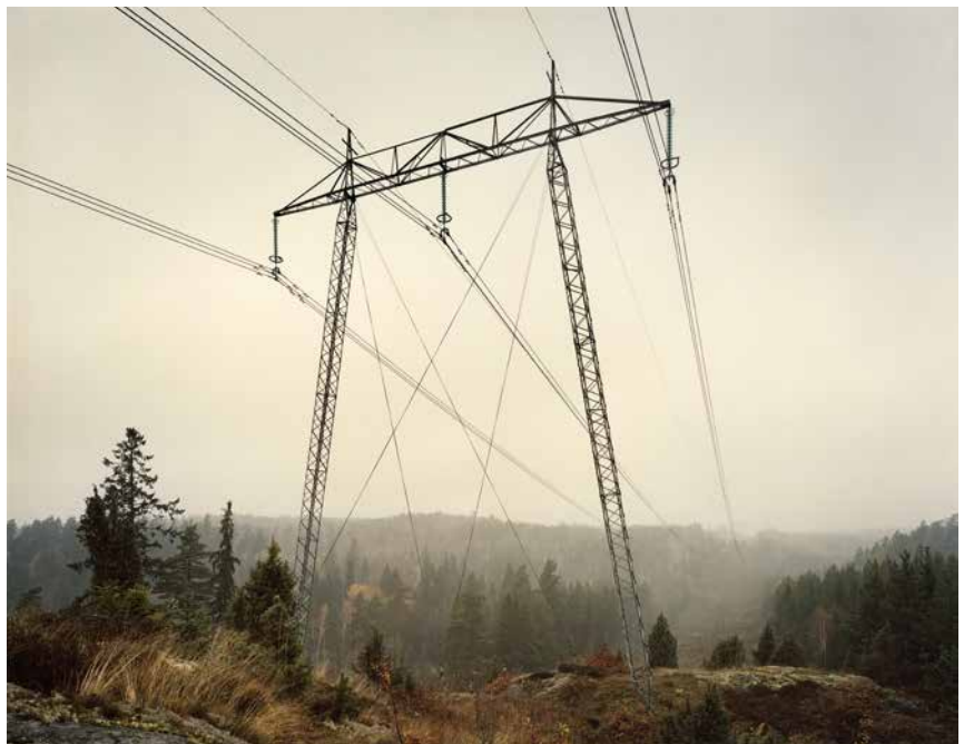
High voltage power line in Sweden.
