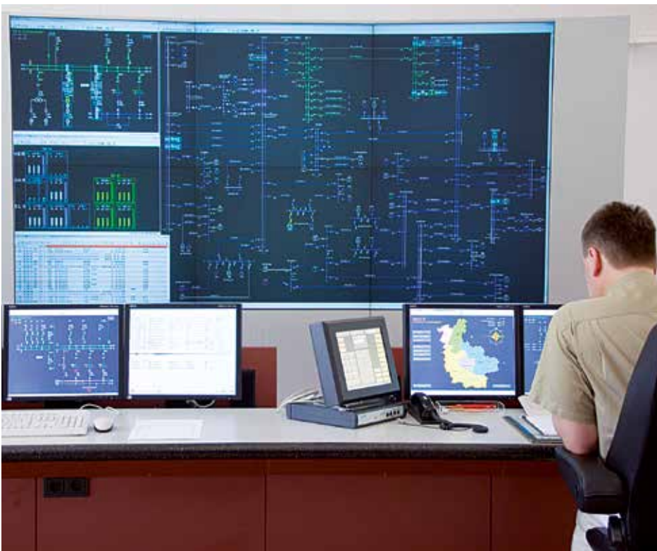
The PSI control system in use at ENERVIE's control center.
