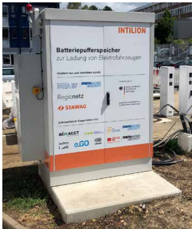
Battery buffer storage for charging electric vehicles.
