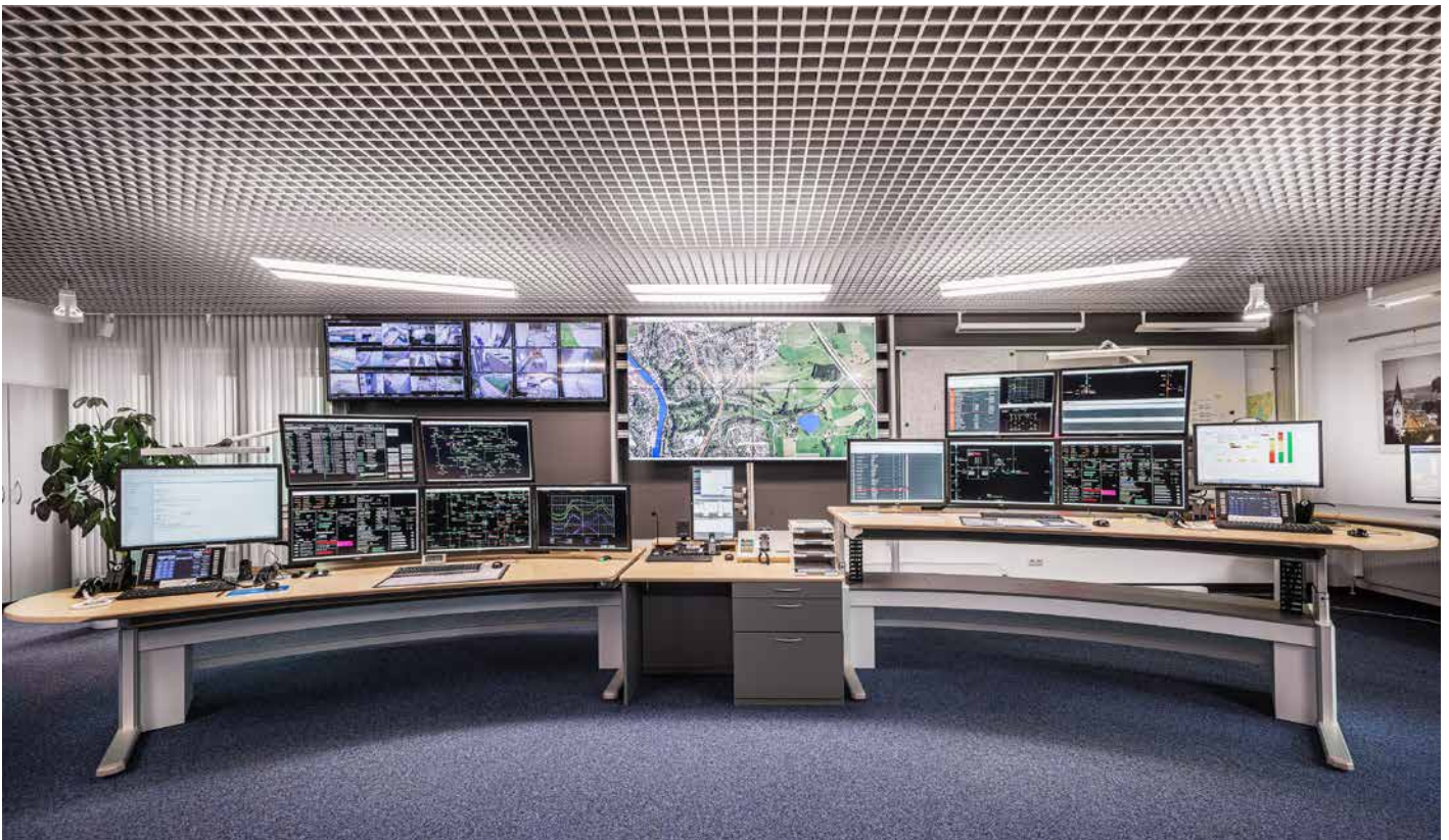
The new control room at AllgäuNetz.
